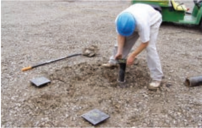
Pre-construction brackets were then placed on each pier. After the installation of the piers, the pad was ready for the remainder of the construction crew to get to work.
