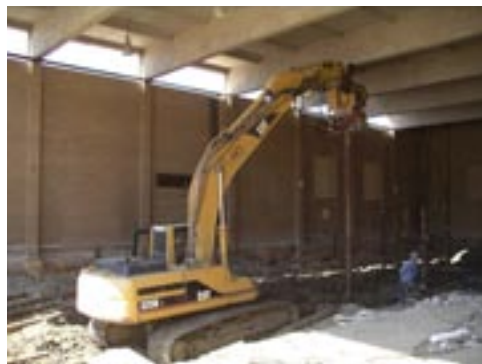
Excavator installs HEATanchors HC Pile Shafts 200 feet deep inside the pool building.
