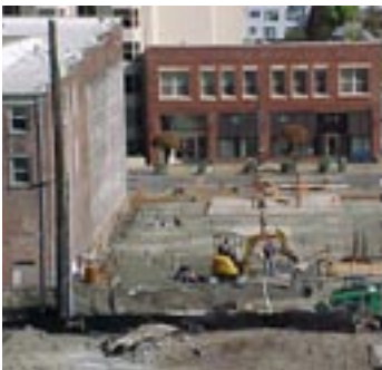
No room for error: HEATanchors vibration free, high capacity pile driven next to aged brick building.
