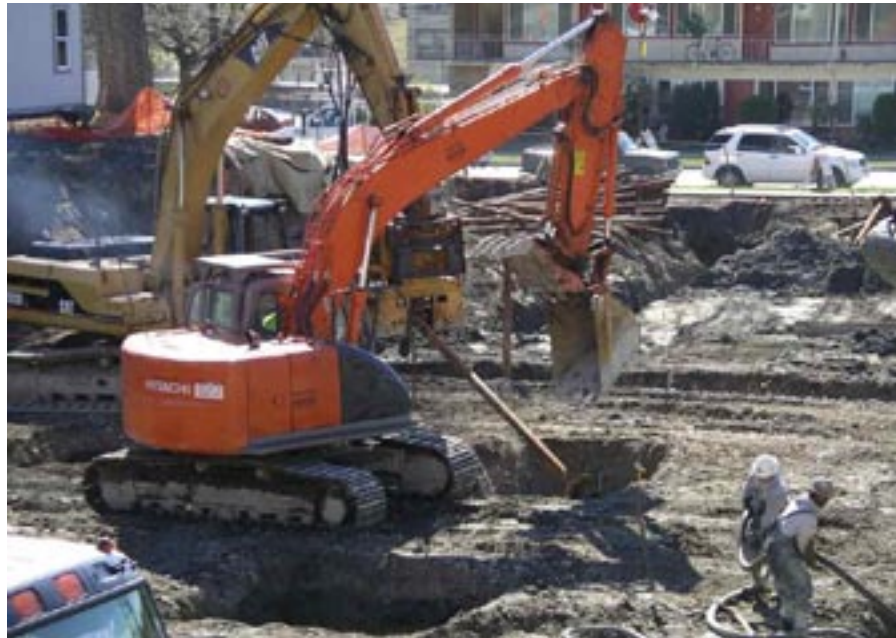
Two workers in excavators install HEATanchors; our job sites are not clogged by unnecessary equipment and manpower.
